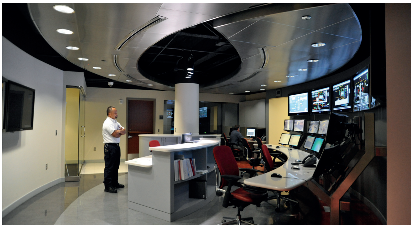
Figure 13: The control room of Thermal Energy Corporation in Houston, Texas, where a recent $377 million energy infrastructure expansion added 48 MW of CHP that operates at 80% efficiency.
