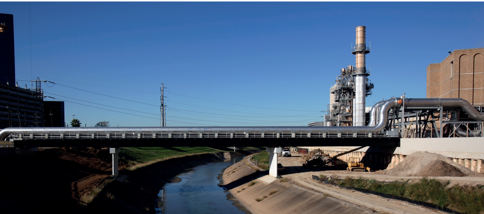
Figure 11: Pipes run over a canal at Thermal Energy Corporation, the district energy company that provides heating and cooling to the Texas Medical Center in Houston, the largest medical center campus in the world.
