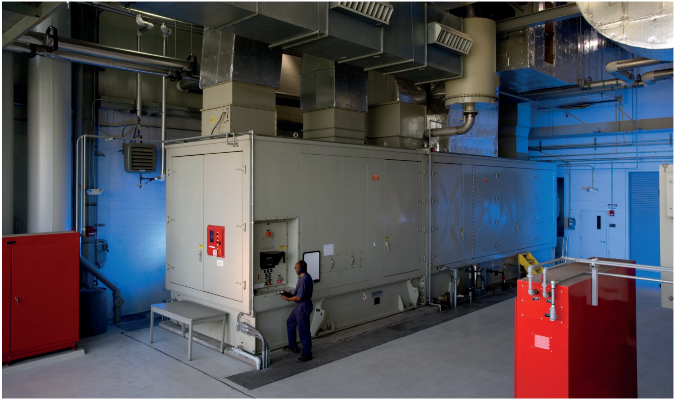
Figure 25: The Central Utility Plant at the University of Cincinnati in Cincinnati, Ohio provides heating, cooling, and power to the University campus and hospital.
