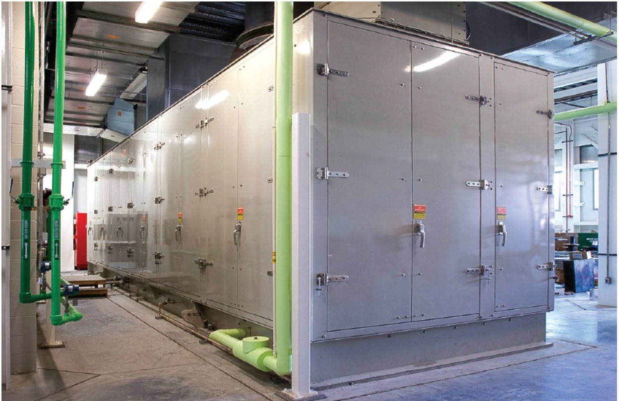
Figure 7: Gainesville Regional Utilities won an Energy Star CHP Award for the South Energy Center, which has an operating efficiency of over 60%.
